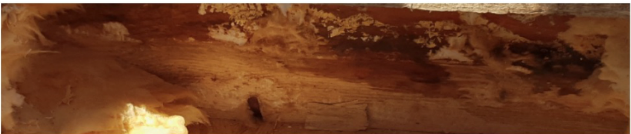
Figure 2 –Signs of deterioration within the built-up
